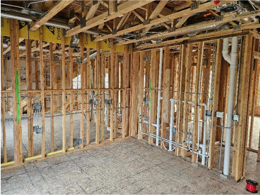
Typical Kitchen wall- Electric, Plumbing, HVAC
