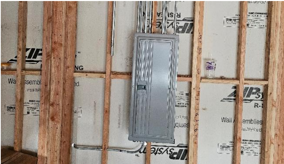
Typical 200amp Service Panel- 8 Units Complete
