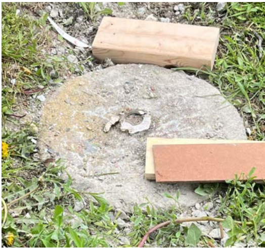
Concrete Tube Base
