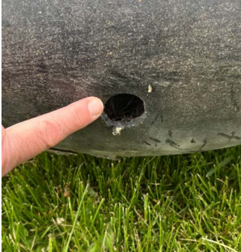
Excessively Large Weep Hole
