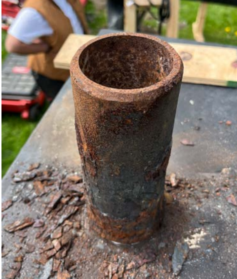
Steel Mounting Pipe on Rectangular Structure
