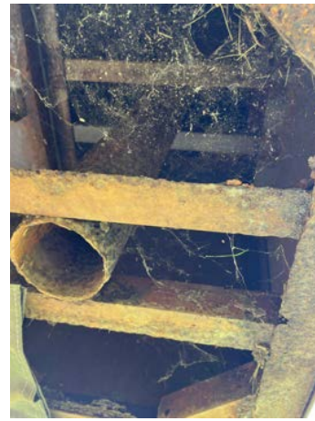
Rusted Angle Iron Interior
